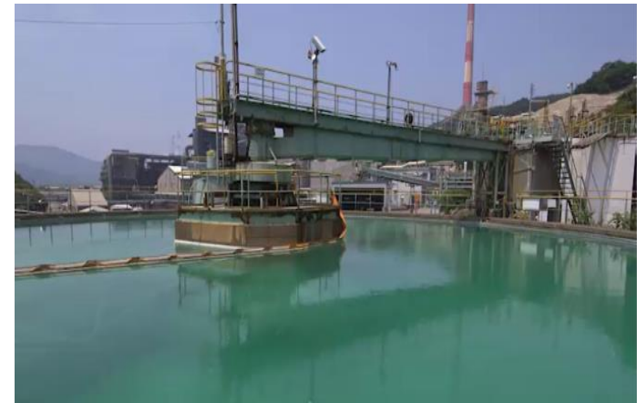
Waste water treatment plant
